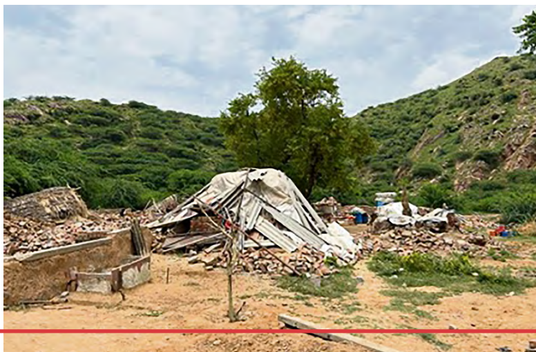
Fig. 1: Homes demolished in Nuh-Mewat after the outbreak of violence between the residents and supporters of vigilante groups. (Photo courtesy of Akram Akhtar Choudhary, 2023)
