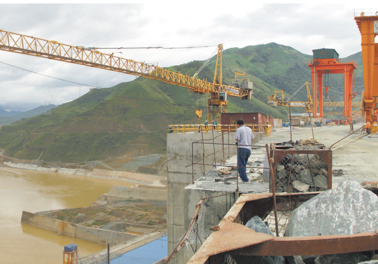
Left: The construction of the Son La hydro-power dam in Northwest Vietnam (© Tuấn CaNon panoramio.com/photo/55081112).
