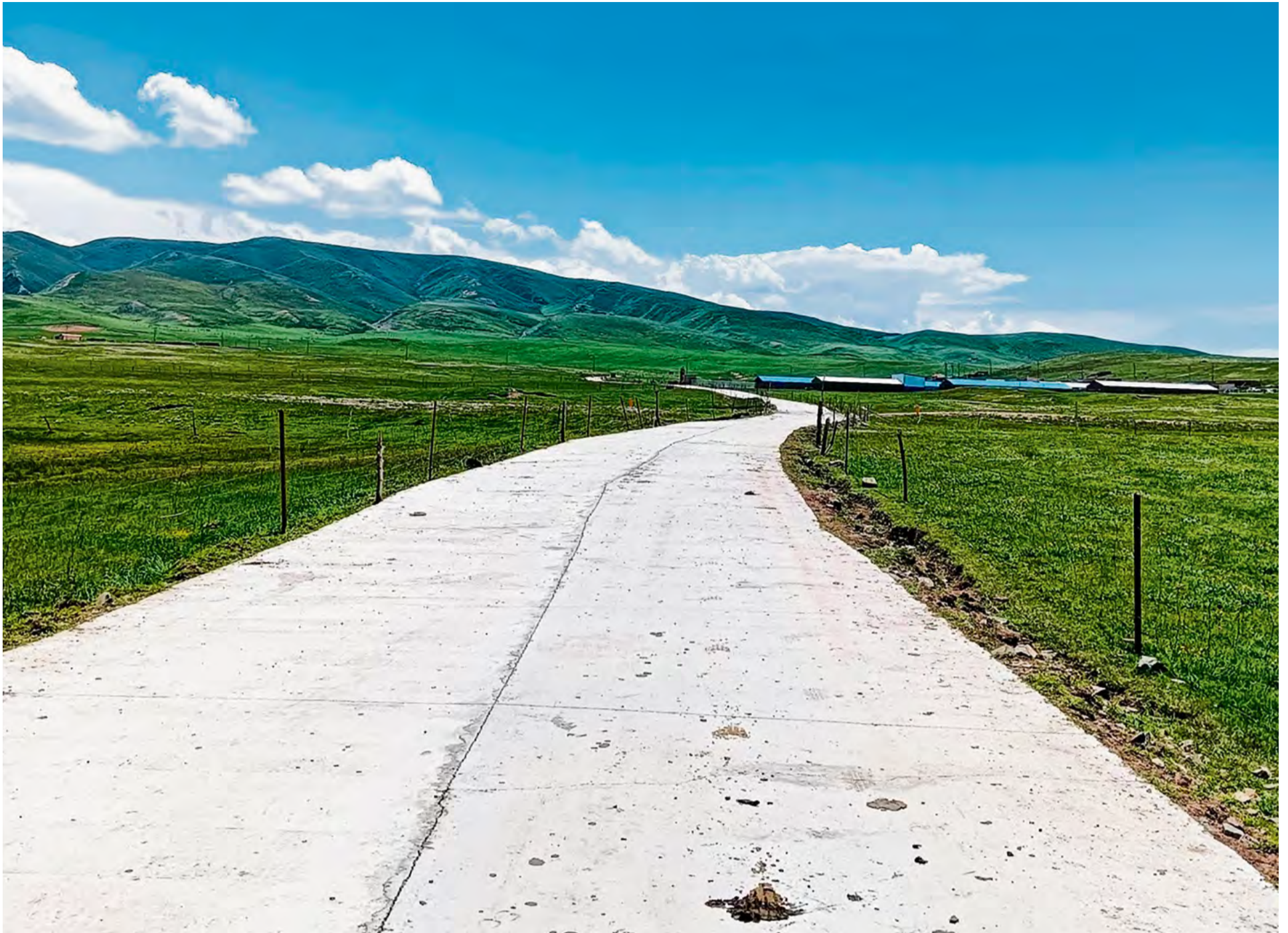
Fig. 2: Part of the new concrete road in Yangden. (Photo courtesy of Gur Gon, 2023)
