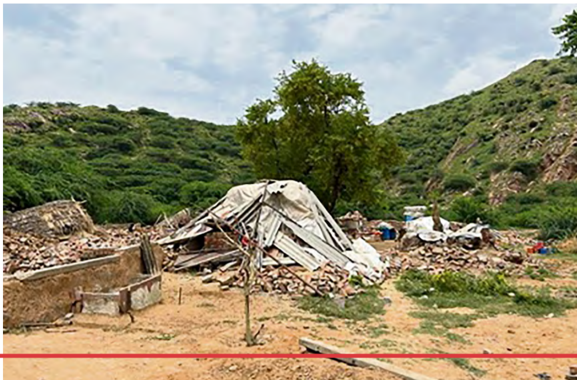
Fig. 1: Homes demolished in Nuh-Mewat after the outbreak of violence between the residents and supporters of vigilante groups. (Photo courtesy of Akram Akhtar Choudhary, 2023)
